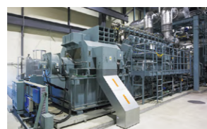
Co-generation system at Tokachi Plant of Meiji Co., Ltd.
