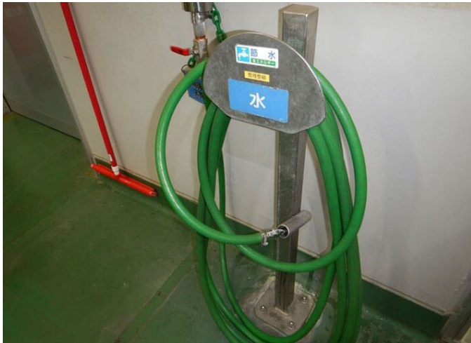
Hose with water-saving nozzle in Asahikawa plant, Meiji
