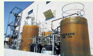
Methane fermentation treatment facility for Meiji Chewing Gum Co., Ltd.
