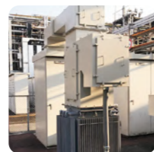
Energy-efficient transformer at Meiji Seika Pharma's Gifu Plant
