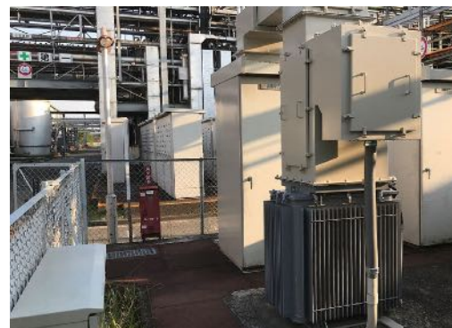
Energy-efficient transformer at Meiji Seika Pharma's Gifu Plant
