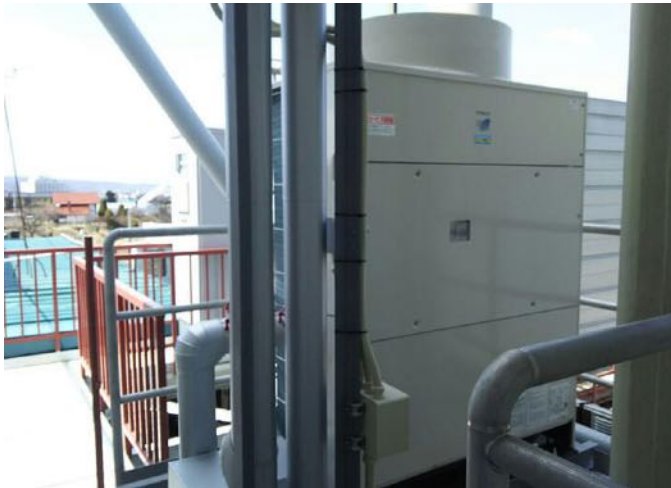
Chillers in Nagano Cheese Plant
