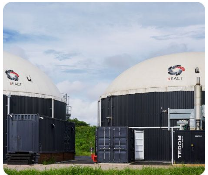
"React Yonezawa" biogas plant with a stylish appearance
