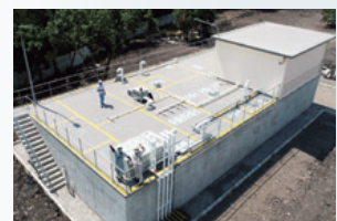
PT. Meiji Indonesian Pharmaceutical Industries' activated sludge treatment system
